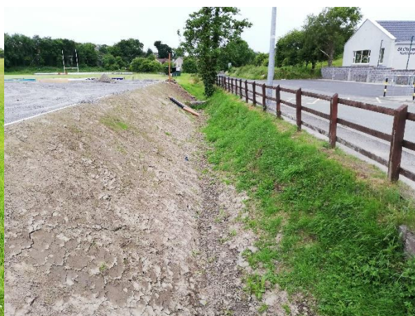
QG4 – Quignamanger, roadside stormwater swale (11 July 2022)
